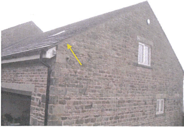
P1 South Gable, gap under end tile
