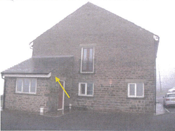
P3 North gable, gap under gutter
